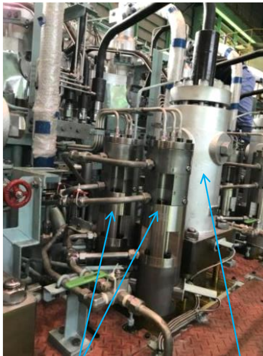
Water injection pump
